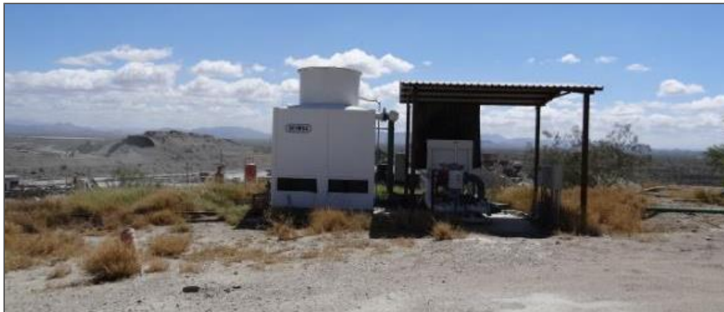
Figure 5.2 View of a Water Well Located on the San Francisco Project
