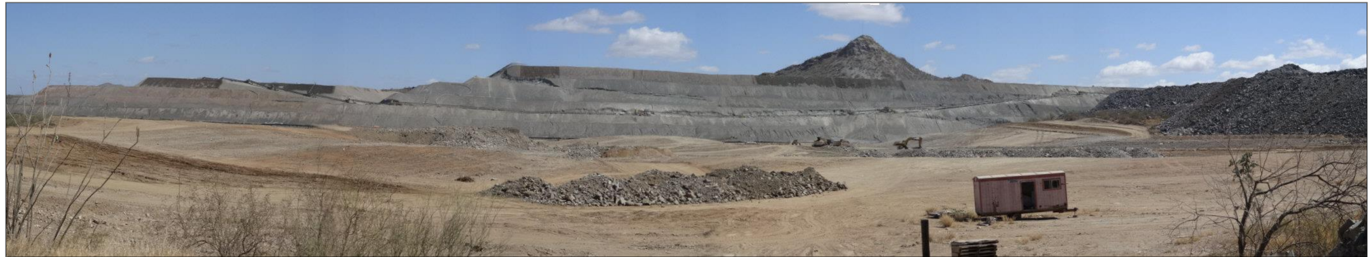
Figure 17.8 Heap Leach Pads as Viewed from the Road to the La Chicharra Pit with Phase 6 Under Construction in the Foreground (May, 2017)
